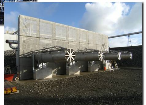
Ladder Heatshields protecting processing piping in KUPE GAS onshore 'Burn Pit'
